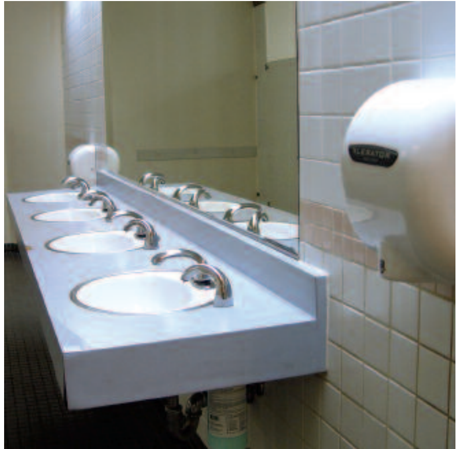
The restrooms in the California State University, Northridge, Student Union utilize Waterless No-Flush urinals and XLERATOR hand dryers as part of the school's commitment to environmental design and water conservation.
