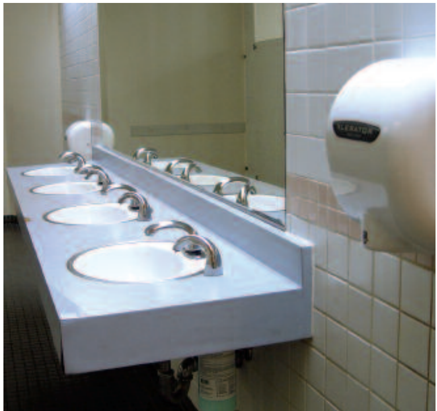
The restrooms in the California State University, Northridge, Student Union utilize Waterless No-Flush urinals and XLERATOR hand dryers as part of the school's commitment to environmental design and water conservation.
